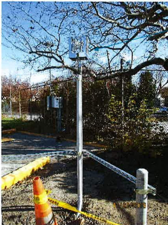
Photograph 2 – Solar powered wet sensor electronic housing
