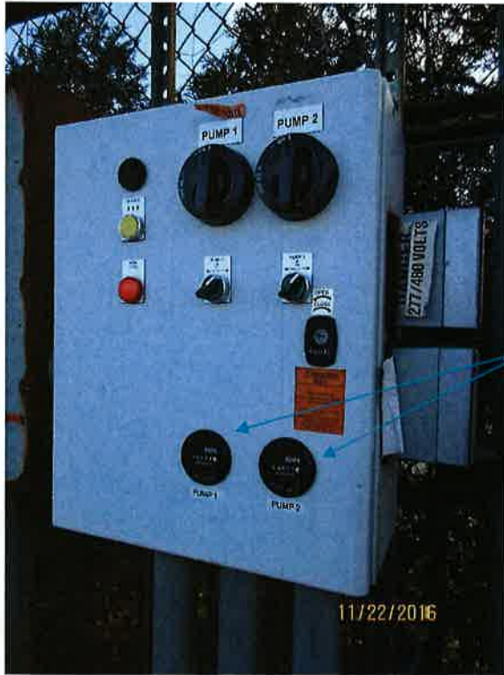
Photograph 1 – Pump run-time meters
