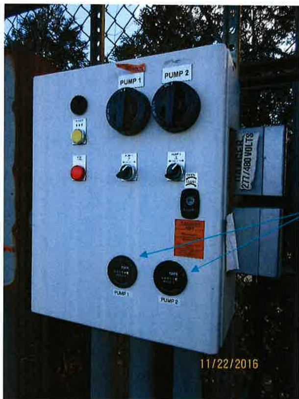
Photograph 1 – Pump run-time meters
